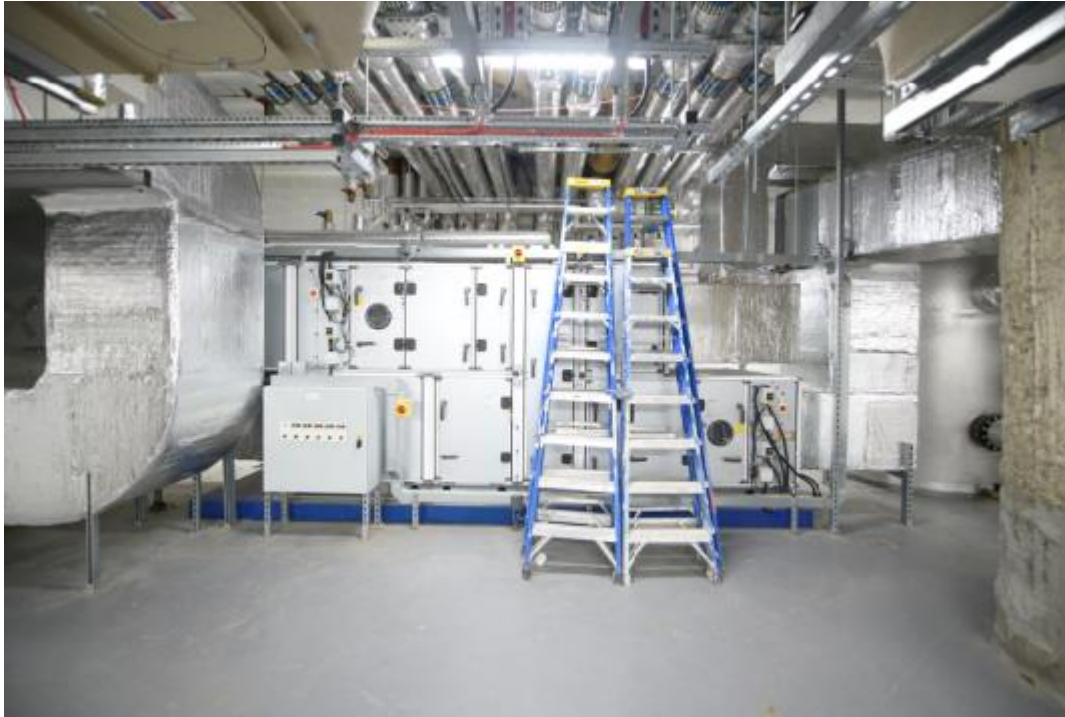
Basement 5 Plant rooms
