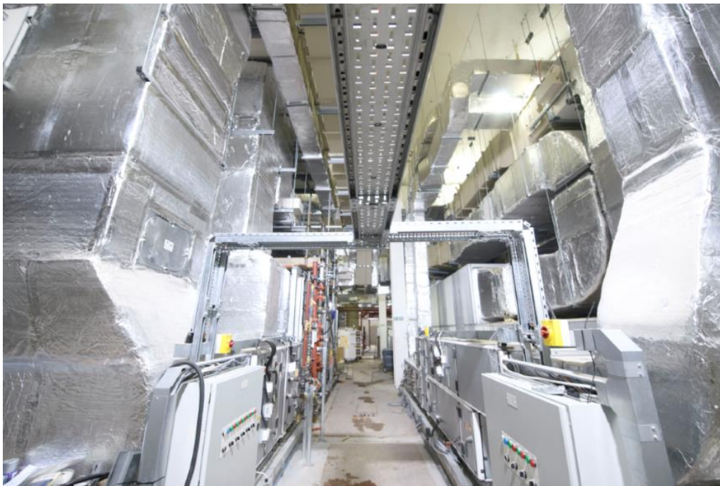
Basement 4 AHU plant room
