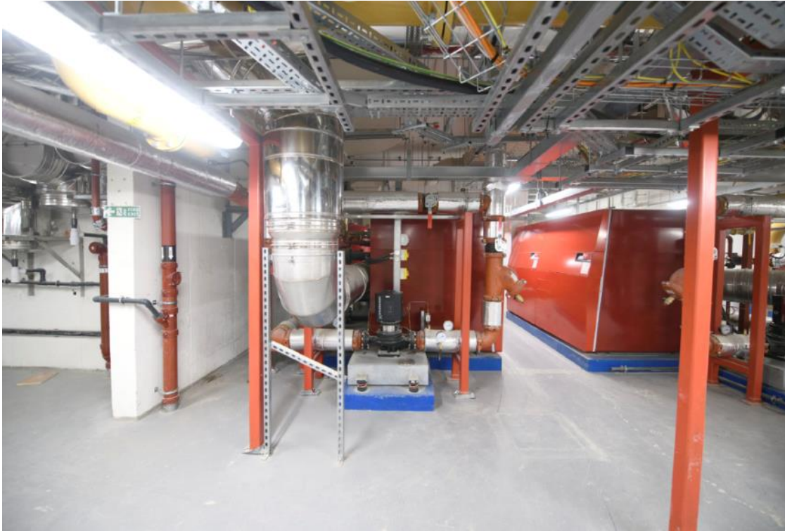
Basement 5 Boiler Plant
